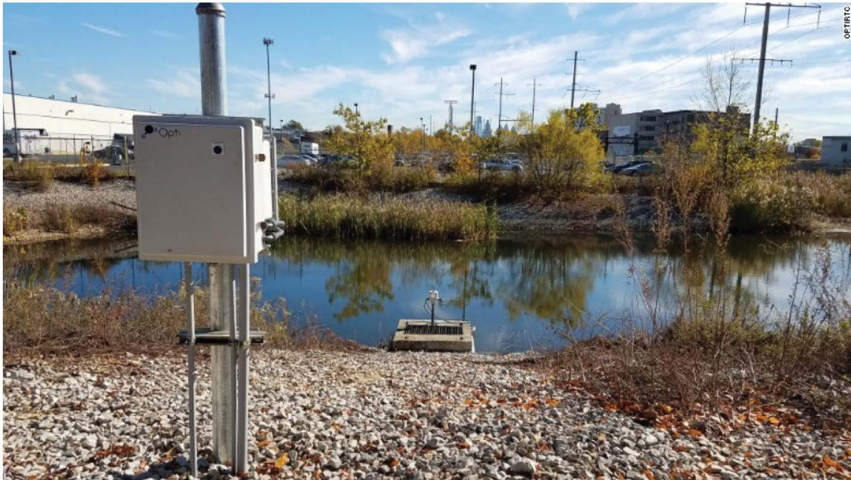
Opti's stormwater management system. Credit: Opti
